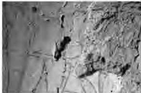
A particularly fragile area where the plaster has lifted from the masonry
